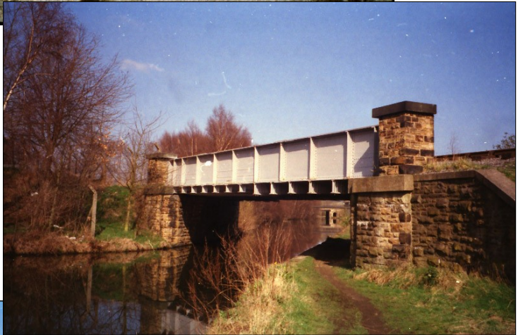
The contro- versial EWS bridge over the Calder and Hebble naviga- tion at Dews- bury
