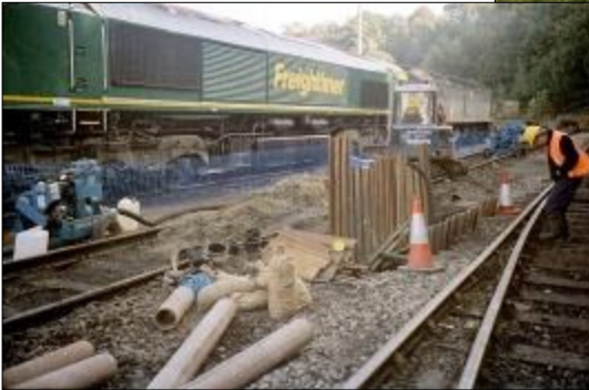
Left, Heavy works going on at Ipswich Fuelling Point to overcome years of pollution.
