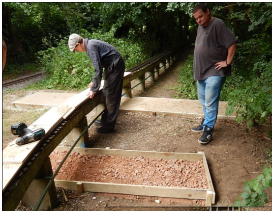
Concrete pads for the raised track point in the woods. One complete in the background and the other two being excavated and form work being constructed.
