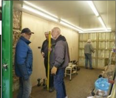
Left top Mike Manners concentrates on the electrical socket outlets in a new wall board
